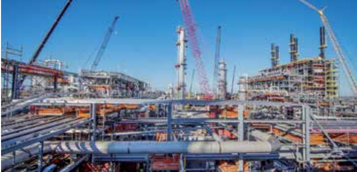
Mechanical contracting and process plant engineering
